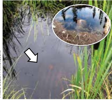
Sunken culverts can block flow.
